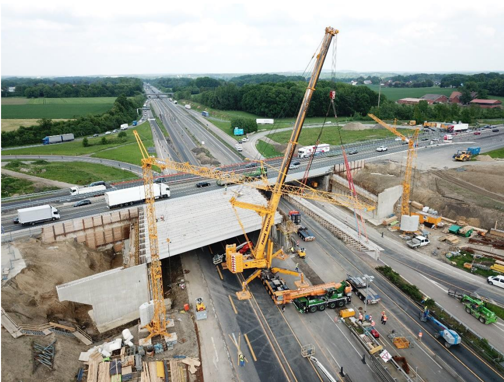
Construction of the temporary bridge at motorway junction Lotte/Osnabrück, © Rekers Betonwerk GmbH & Co. KG
