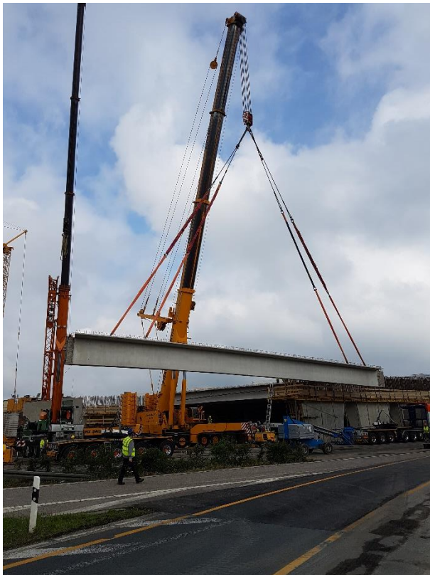
Prestressed concrete beams measuring 36 metres in length. The precast unit formwork was constructed using 24 alkus ® AL 20 panels with a total surface area measuring over 200 square metres. © Rekers Betonwerk GmbH & Co. KG
