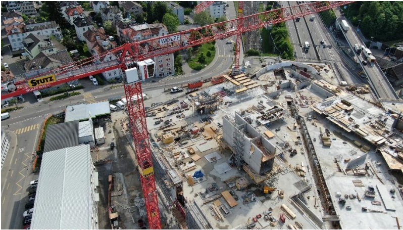
The construction site: The new hall 1 is under construction in St. Gallen. | © alkus AG
