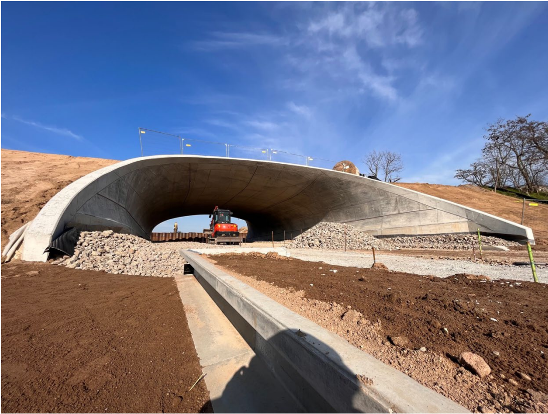
The 40-metre-long tunnel above the bicycle highway on the BUGA 23 site was designed as an open-cut construction. | © Kiefer Schalungsbau GmbH
