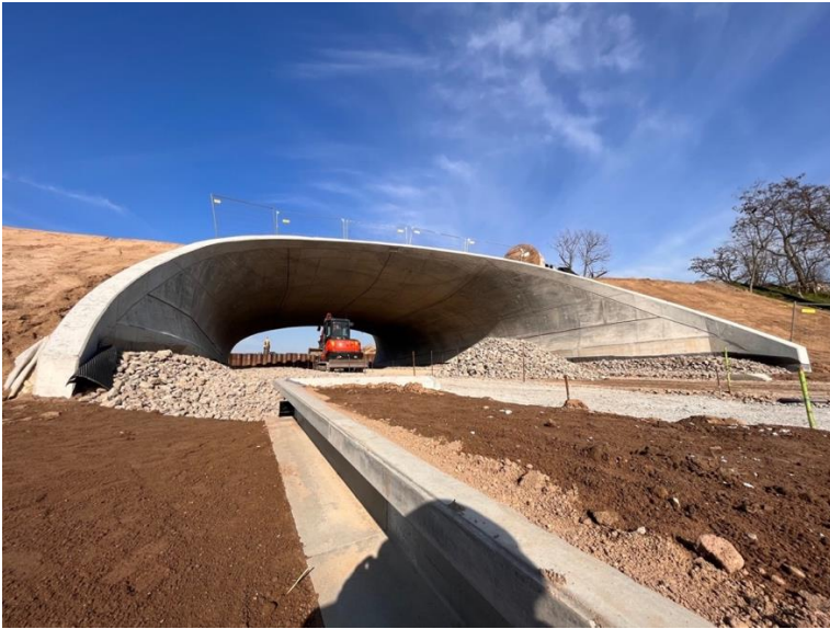
The 40-metre-long tunnel over the high-speed cycle path on the BUGA 23 site was built using the cut-and-cover method. | © Kiefer Schalungsbau GmbH
