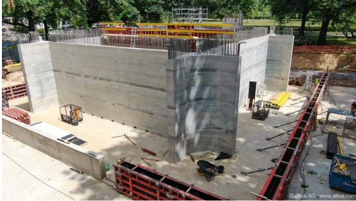
During the construction of the ABMC visitor center in Margraten, the alkus ® formwork panel ensures a smooth concrete surface without gaps or holes. | © alkus AG
